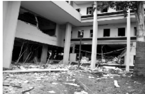
Figure 7: UN office bombed in Abuja, Nigeria (source- Photo News 3)
